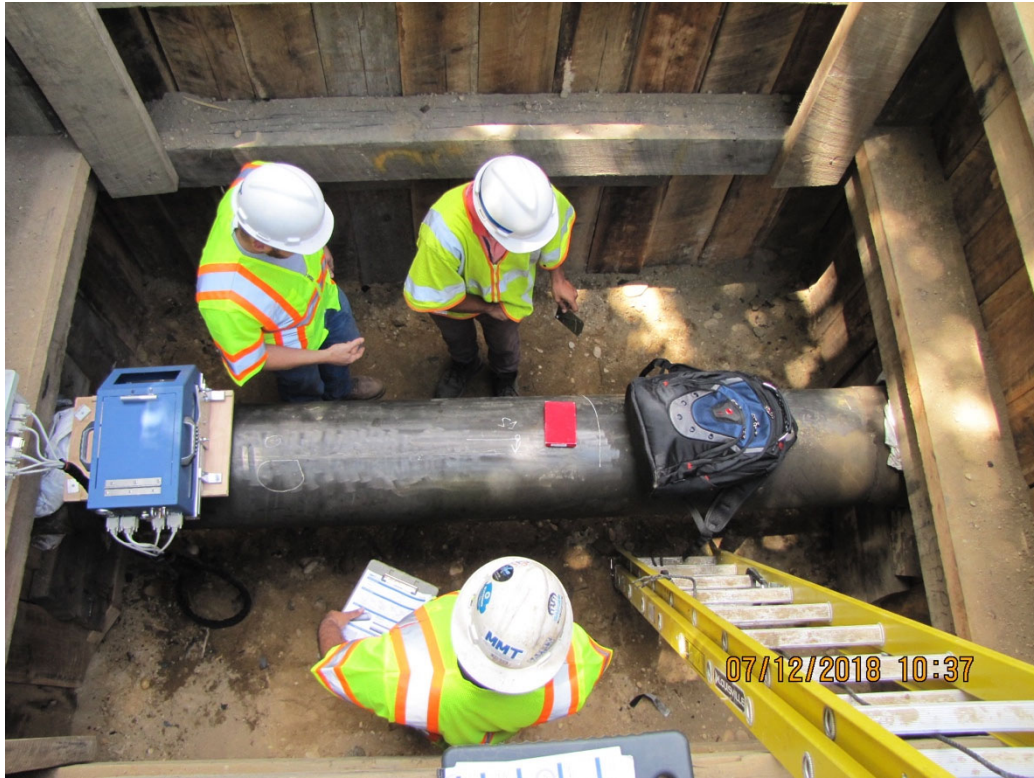
Fig. 12: In-ditch assessment utilizing the HSD Tester and NDE methodology for longitudinal seam verification.
